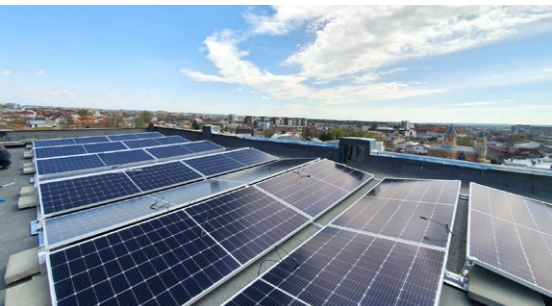
Solar panels installation in progress on a technical building of our customer - Romania
