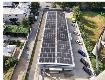
Solar system on rooftop of a technical building, Aktivco's SaaS project - Romania
